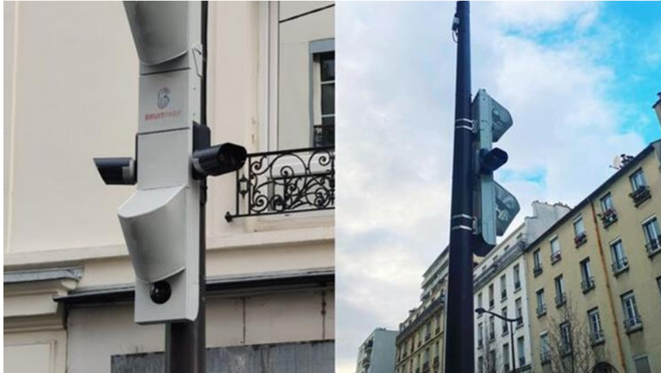
The noise radar has been installed high on a street lamp post in the 20th district in eastern Paris. (@David_Belliard/Twitter)
